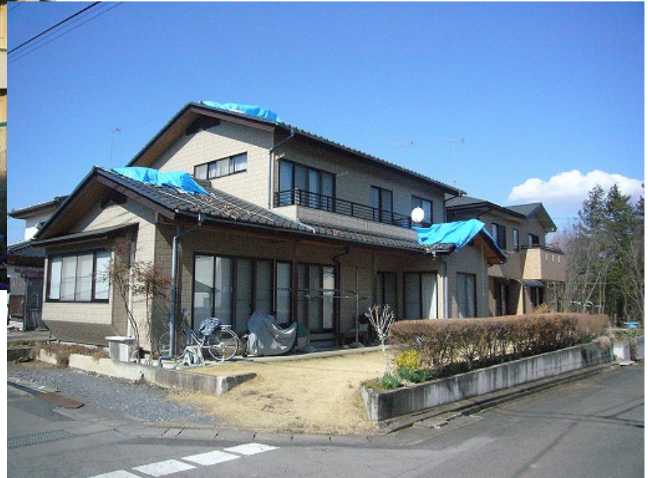
Several houses have damage in the roof around TCGH16, 1.2g site.
