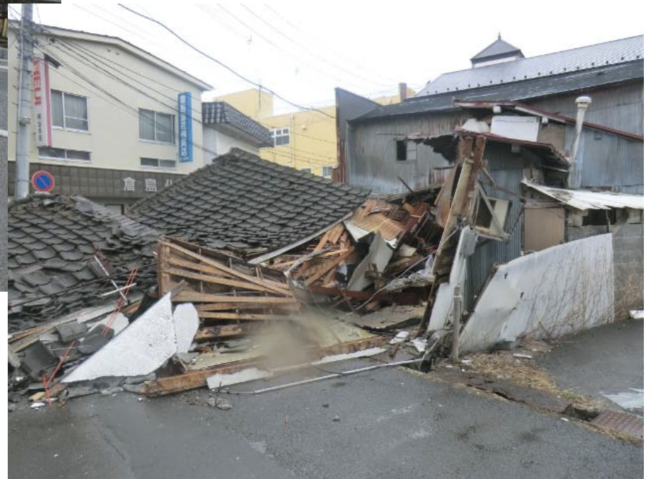
Several wooden houses collapsed around MYG006, JMA intensity 6+ site.
