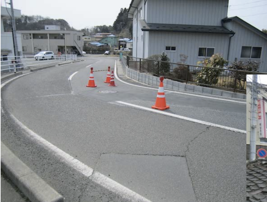
Virtually no severe damage around MYG004, 2.7g site.
