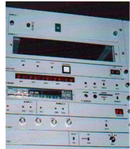
A data logger system
